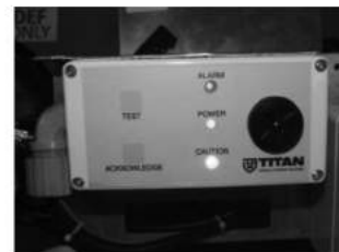
Audible Overfill Alarm
